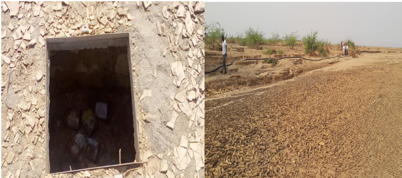
Figure 4.4.1.3: Control chambers for the kiosks filled with dirt and mud in Lughaya transmission pipe wiped away by the floods
