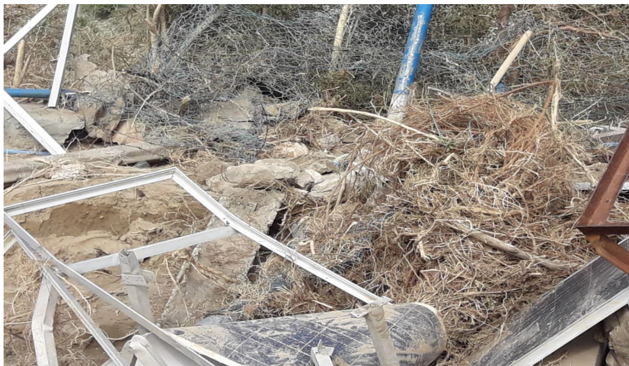
Figure 4.4.1.4: Garbodadar shallow well and solar system wiped away by the floods
